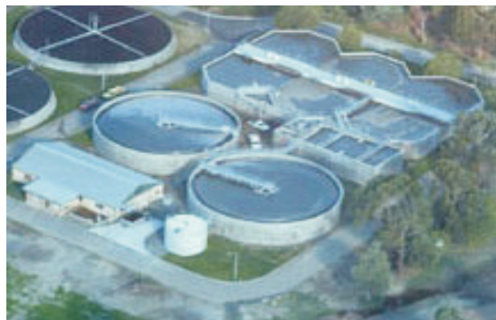
Figure 8.7 An aerial view of a sewage plant
